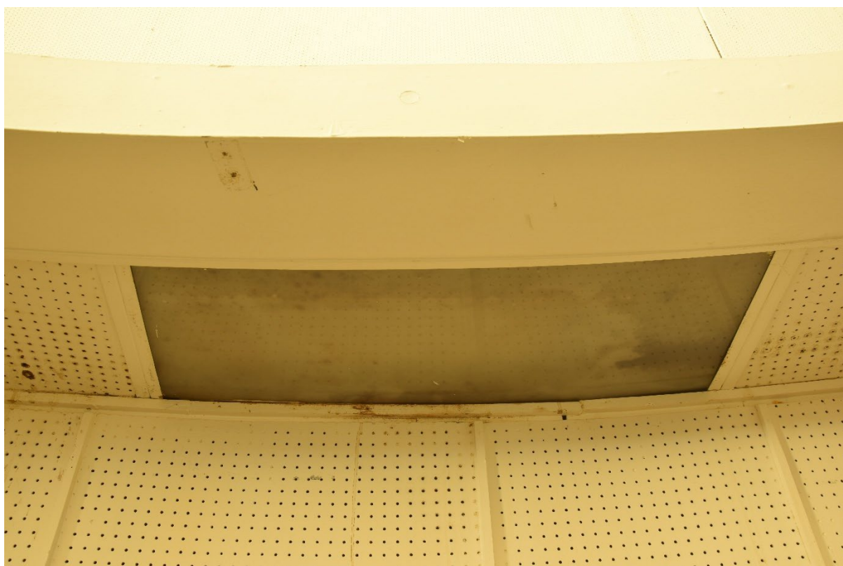
Photograph 54 (below): Down-lighting set into the gutter, looking west
